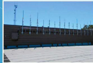
Survivable port entry & mounting system for rooftop antennae array. Boone County, Mo. Emergency Communications Center.
