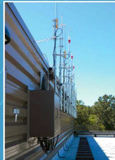
Side view of survivable port entry & mounting system for rooftop antennae array. Note roof membrane walk pad protection. Boone County, Mo. Emergency Communications Center.
