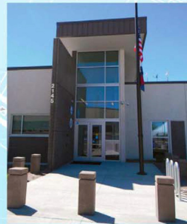
High wind & impact resistant glazing system at building entry. Boone County, Mo. Emergency Communications Center.
