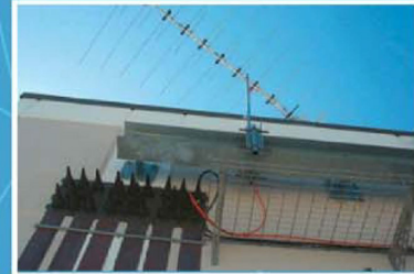
Wall mounted port entry & antennae mounting beam. Sunrise, Fla. Public Safety Building.
