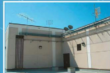
Grounding and wall mounted port entry & antennae mounting beams. Sunrise, Fla. Public Safety Building.
