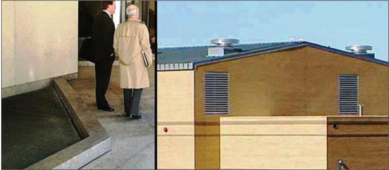
Figure 4-2: A vulnerable, ground-level intake (left); an intake elevated to the second story (right)
