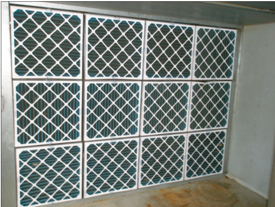
Figure 4-8: A bank of pleated MERV 8 pre-filters in front of MERV 14 cartridge filters in an office building air-handling unit
